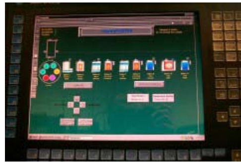
Photo 14 overall view of all 9 stations status
