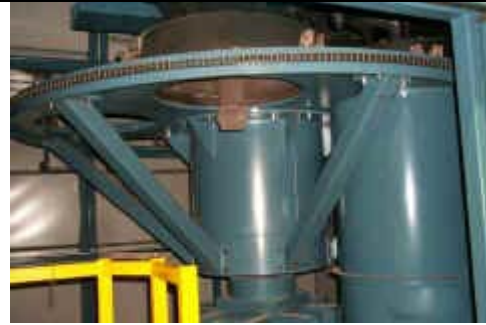
Photo 8 six station load carousel transporter.
