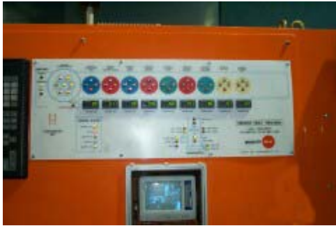
Photo 11 bed monitoring panel
